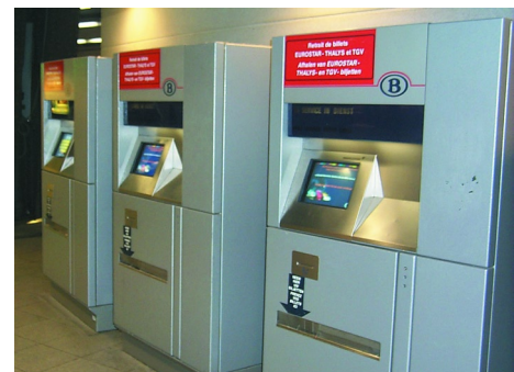
TOD Automatic Ticket Distributor
